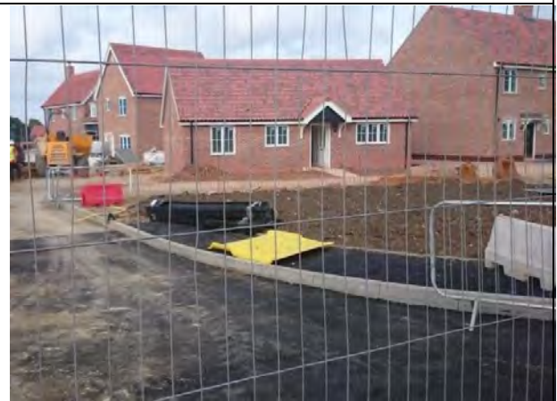
2018 development of 73 new homes on Saham Road just to south of the Parish boundary
