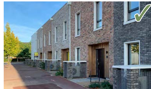
Air Source Heat Pumps are positioned at the front of dwellings to enable easy servicing, but are enclosed to screen them and avoid dominance when viewed from the street.
