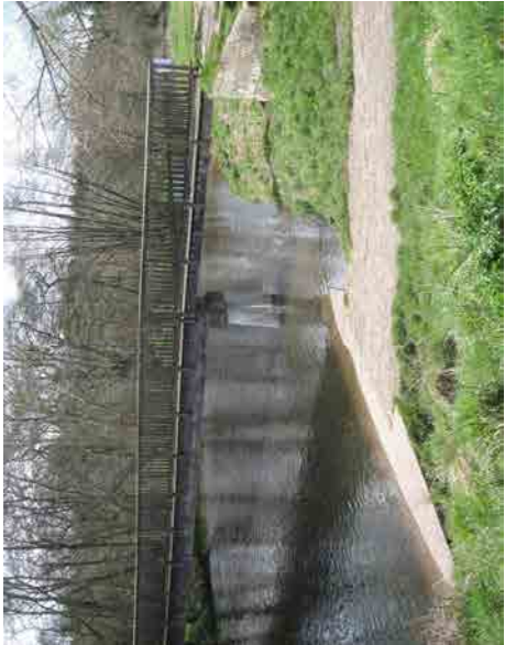
Existing St. Helen's Footbridge carrying the St. Edmund's Way and slipway. The bridge deck requires replacement due to rotten planks.
