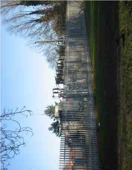
Screen electricity sub station opposite entrance to Thetford Priory.
