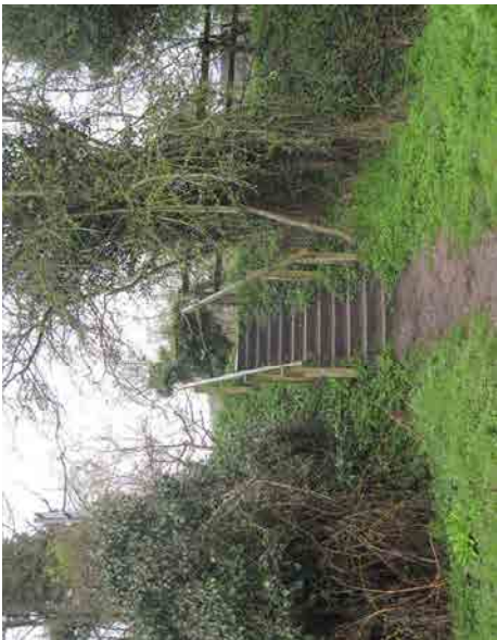
Access point onto the Little Ouse path to St. Helen's picnic area should be redesigned to ensure it is DDA compliant.
