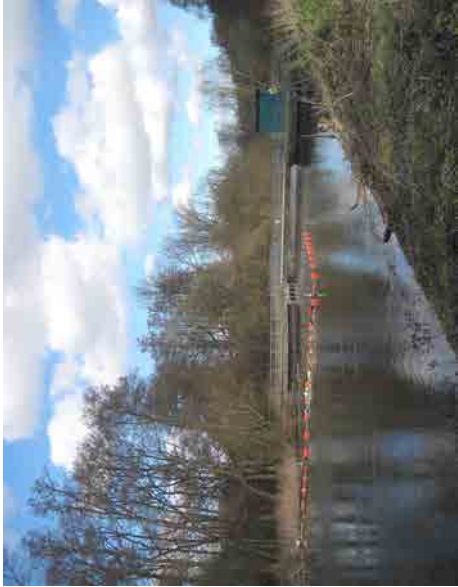
Abbey Heath Weir, the boom would appear to be broken. The weir is very dangerous and should never be attempted by canoeists due to the low headroom beneath the footbridge.
