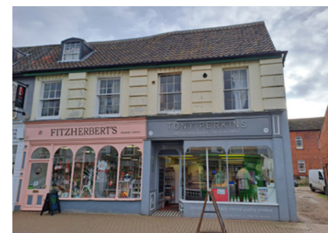
Shopfronts in good condition but first floor neglected with windows and paintwork in poor condition
