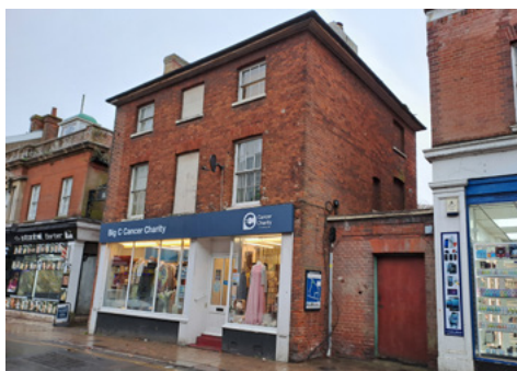
Fascia overly large and windowsills above in poor condition
