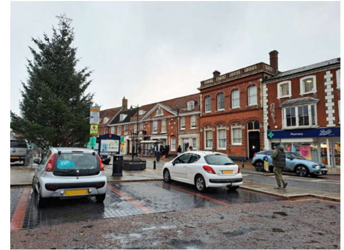
Parking in the Market Place with tarmac in poor condition
