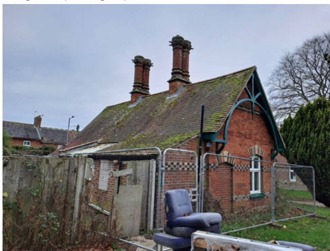
Cemetery building in poor repair with an air of abandonment
