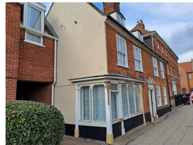
Example of a shopfront likely inserted into a former house, now back in use as a house with shopfront retained at south end of High Street. This shopfront was undergoing repairs at the time of survey.
