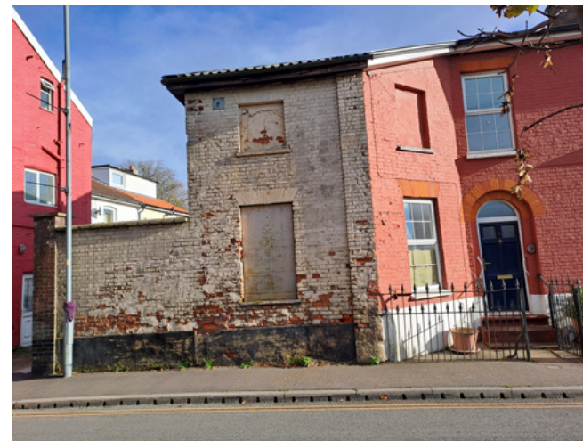
Flaking paint and crumbling brickwork on apparently vacant house on Commercial Road
