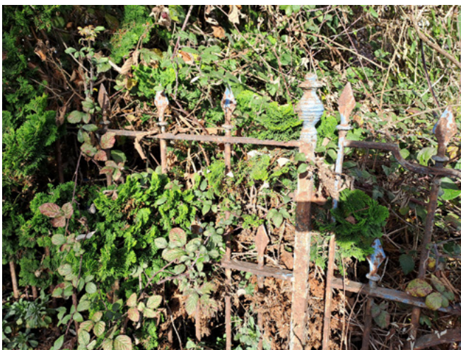
Railings in poor repair on Norwich Street
