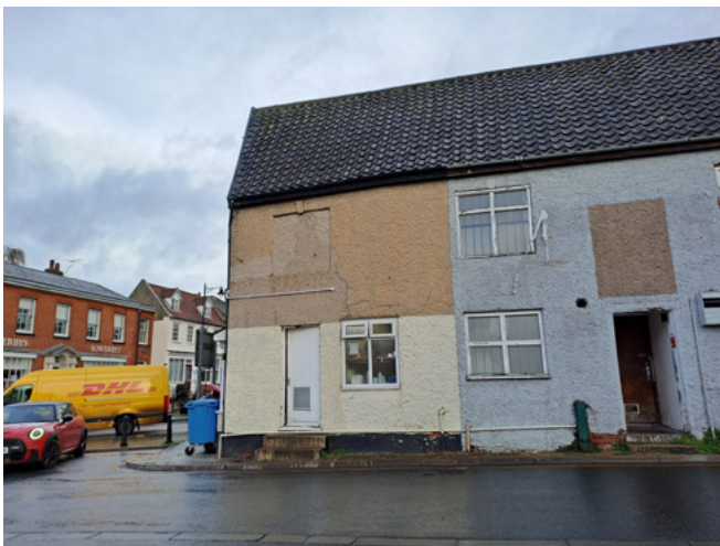
Buildings in poor condition on Quebec Street with cracked render and peeling paintwork to timber windows
