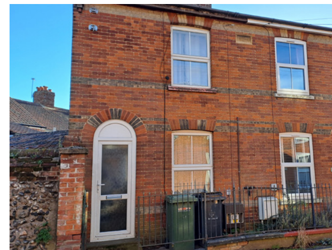
Inappropriate uPVC windows and doors eroding the historic character of both houses
