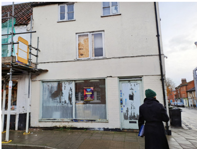
Vacant building on Ruthen place with shopfront in poor condition and generally looking very run-down
